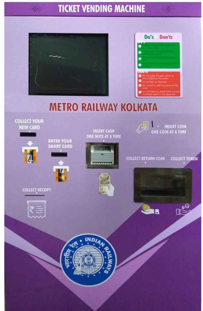
TVM being used by Kolkata Metro at stations for purchasing and recharging Smart Card and issuing of Smart Tokens
